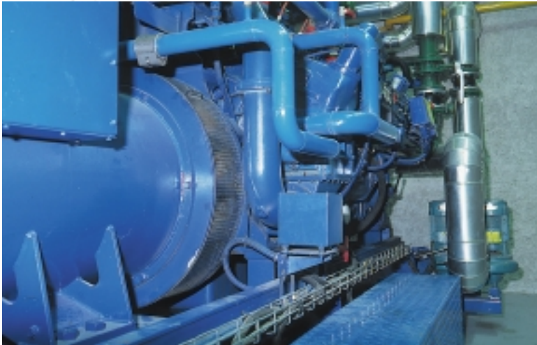
Example of application: boiler plant
